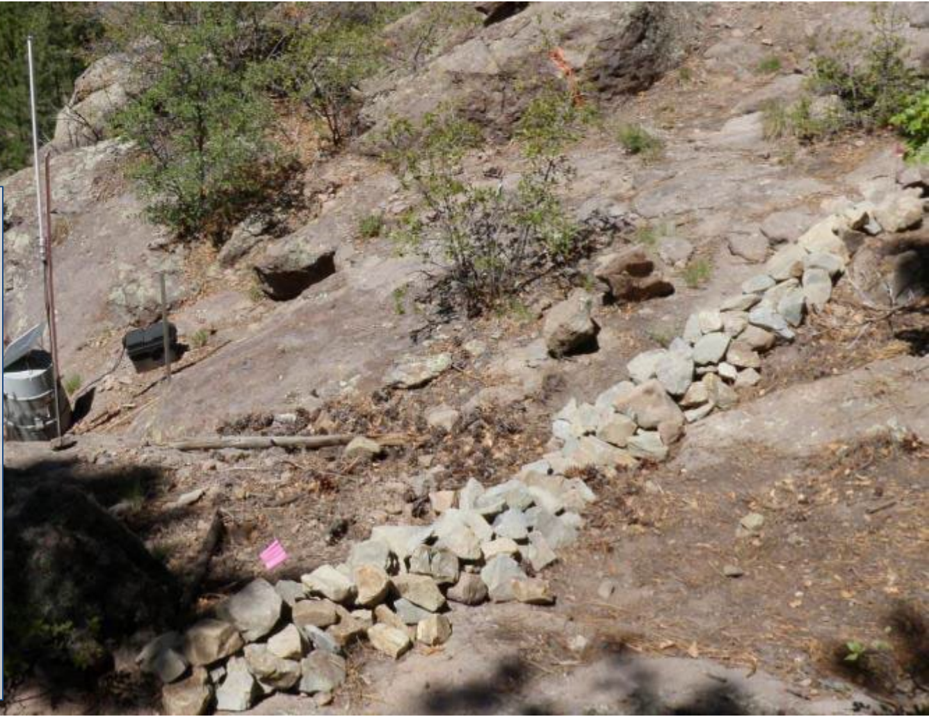
Rock check dam J01006010027 and sampler at PJ-SMA-9.02.
